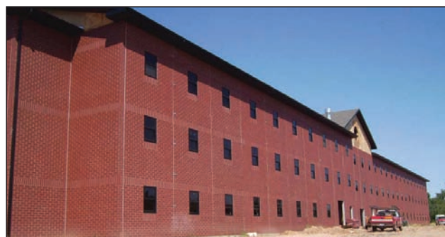
Walton Construction is providing design/build services for the U.S. Army Corps of Engineers' development of the LEED-certified Fort Riley Custer Hill Barracks in Fort Riley, Kansas.
